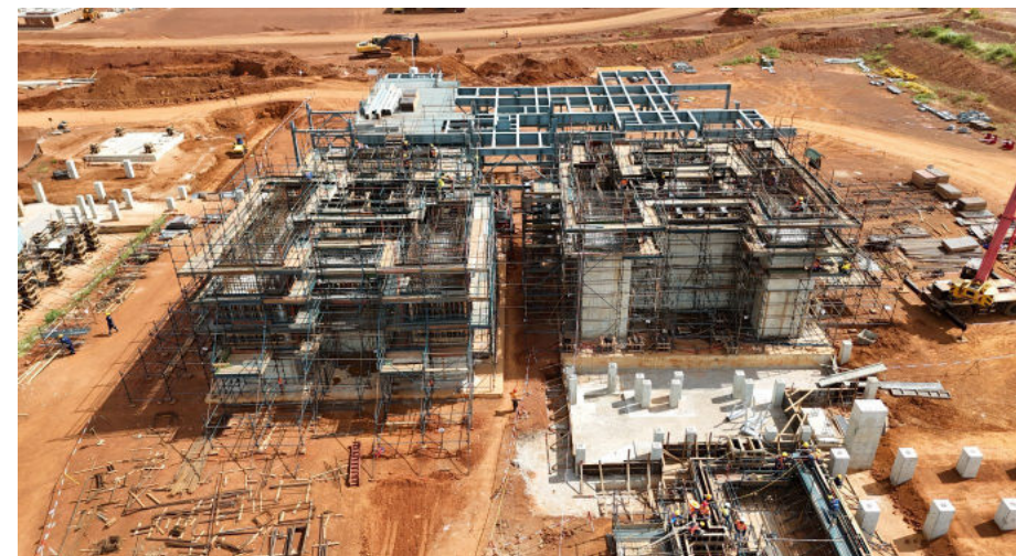
Process Plant- Grinding Area
